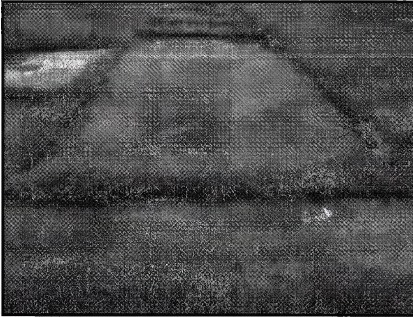
Lot C-51 Standing Water: Observed standing water on the empty pad.
