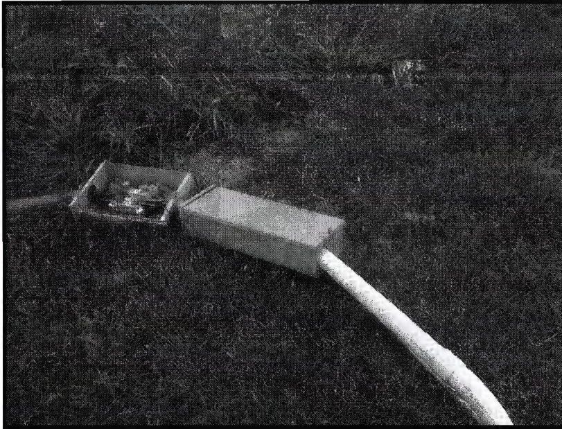
Lot C-48 – Electrical: Observed an electric meter box laying on the ground.
