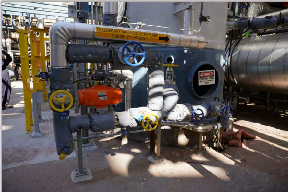
Figure 32. Toledo Refinery Fuel Gas Mix Drum with modifications made after the September 20, 2022, incident. (Credit: CSB)
