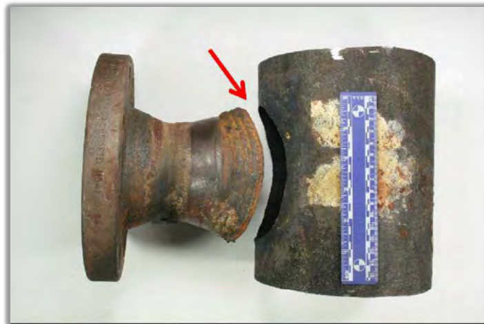
Figure A1-1. Failed branch fitting from the BP Whiting Refinery. (Credit: BP)
